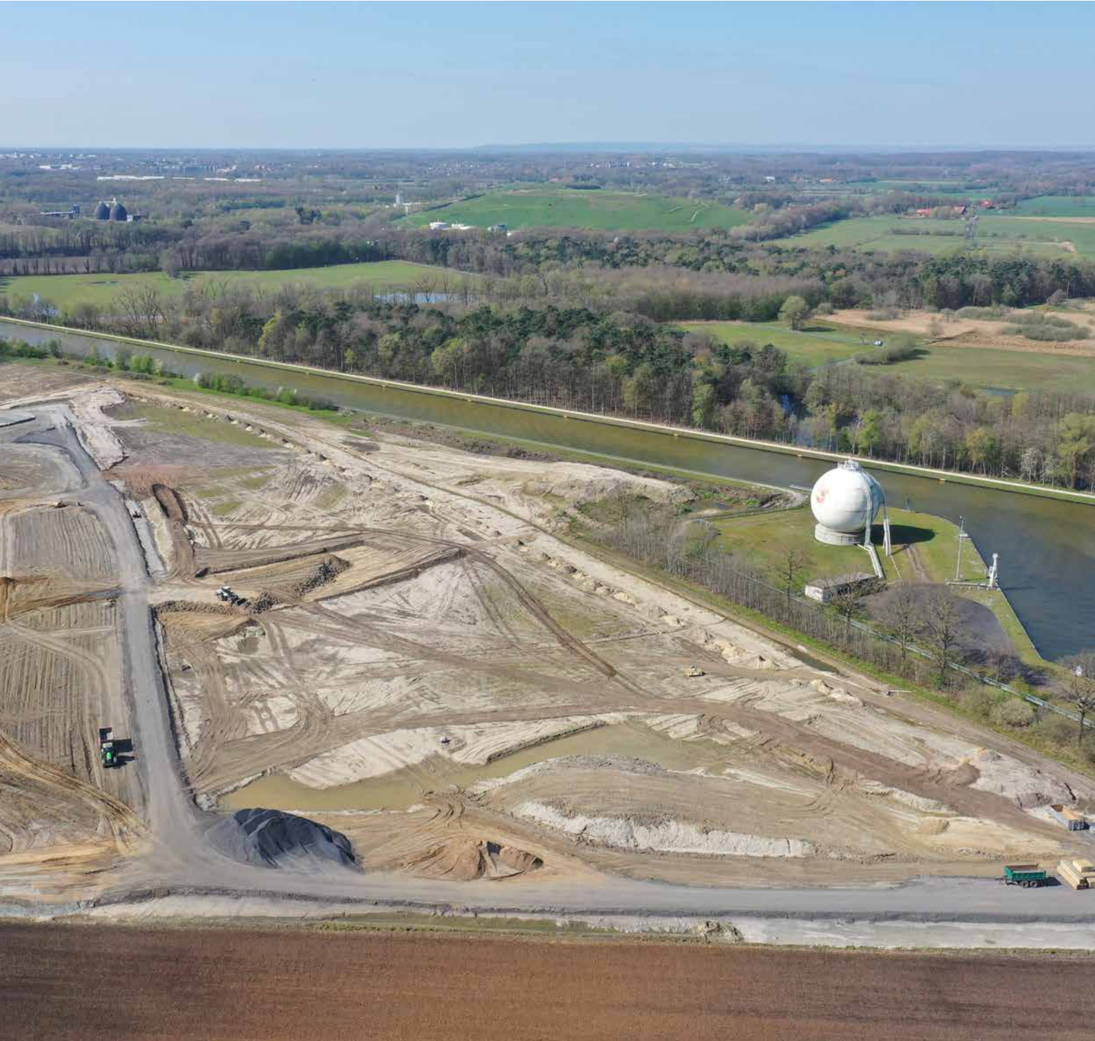
Just one of the site expansion projects: as part of the 'Next Level' initiative, a new filling and logistics site is being built alongside the existing Westfalen tank depot in the port of Münster-Gelmer.
