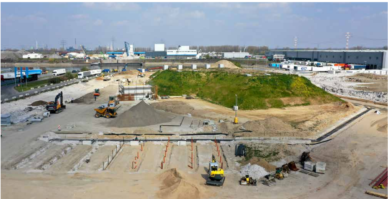
Construction work at the Westfalen Group's Krefeld port site continues apace – grass is already growing on the soil covering the tanks.
